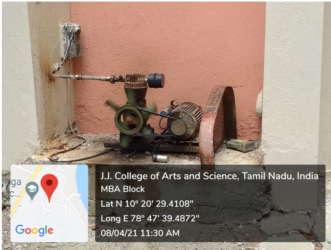
BORE WELL MOTOR (MBA BLOCK)
