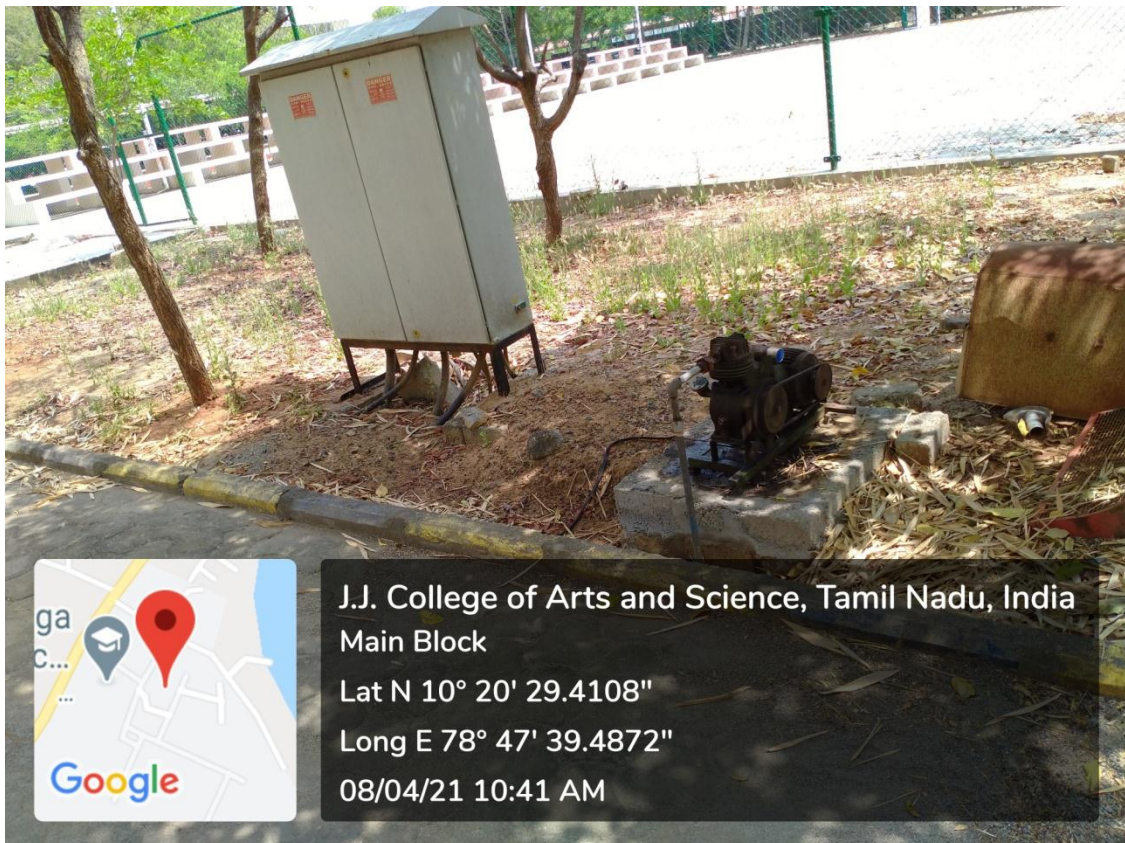
OPEN WELL MOTOR (MAIN BLOCK)
